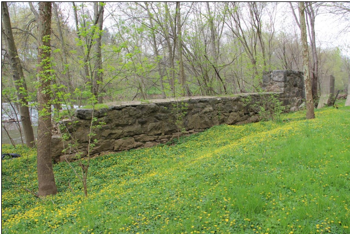
Photograph 8: Detail, Lock No. 5 showing west wall of lock, altered and reincorporated into twentieth century hydroelectric dam (demolished) and sluice gates, facing northwest.
