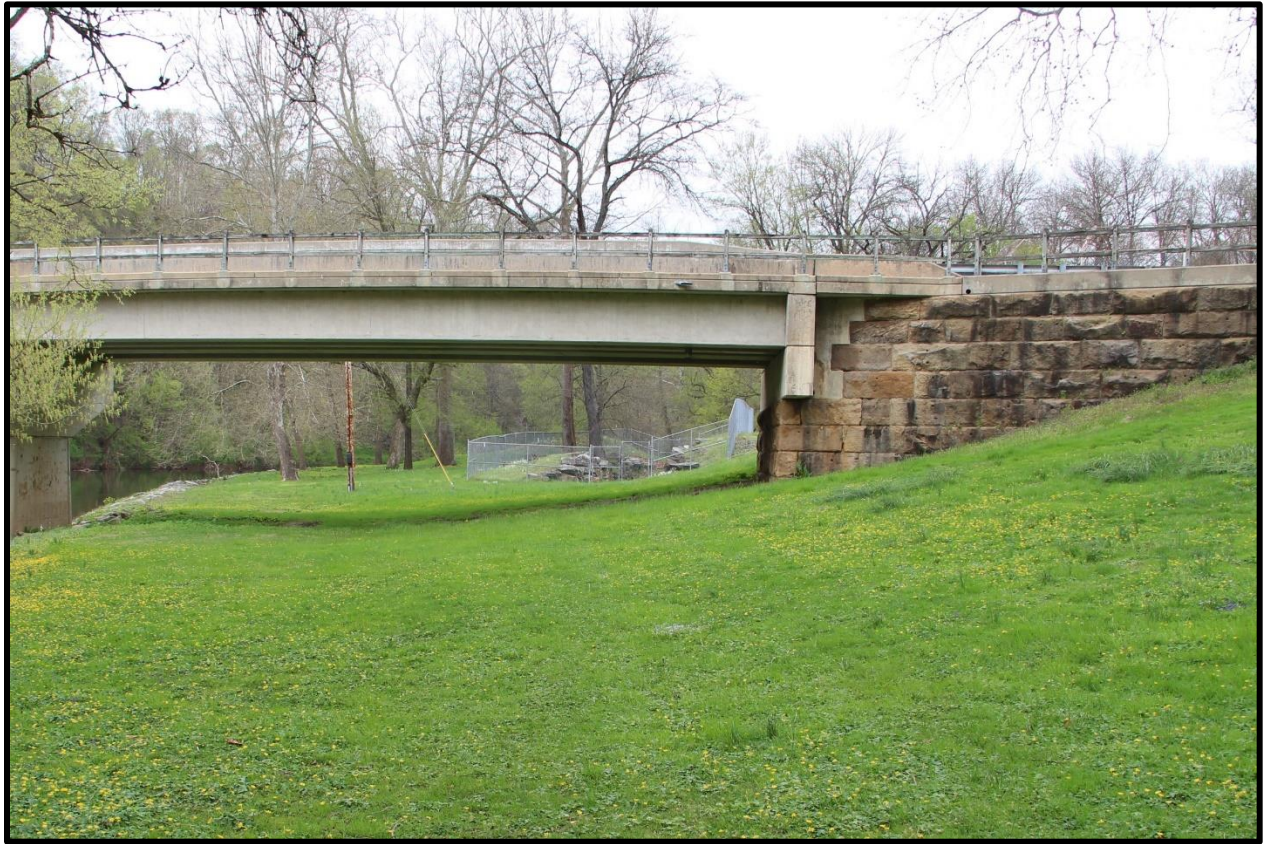
Photo 5: Overview, Conestoga Canal Lock No. 6 showing relationship to River Road (SR 3017) Bridge and abutment. View from southern side of River Road Bridge, facing north.
