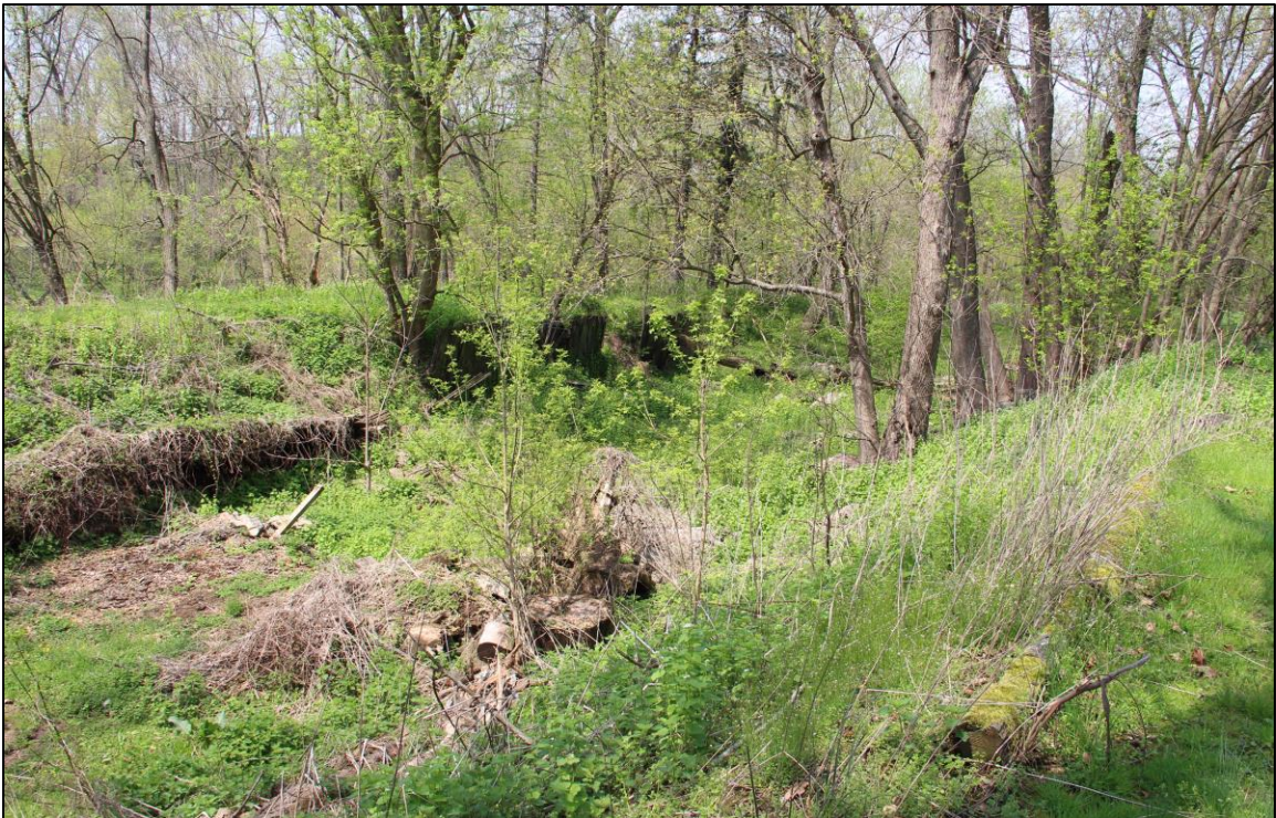
Photograph 14: Detail, Lock No. 4 sluiceway, facing north. Age and association of wooden features (middle) are unknown.
