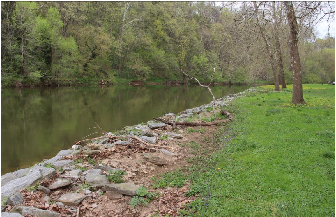
Photograph 2: Detail, east embankment of Conestoga River, showing rip rap, west of Lock No. 6 (Lock No. 8), facing northwest.
