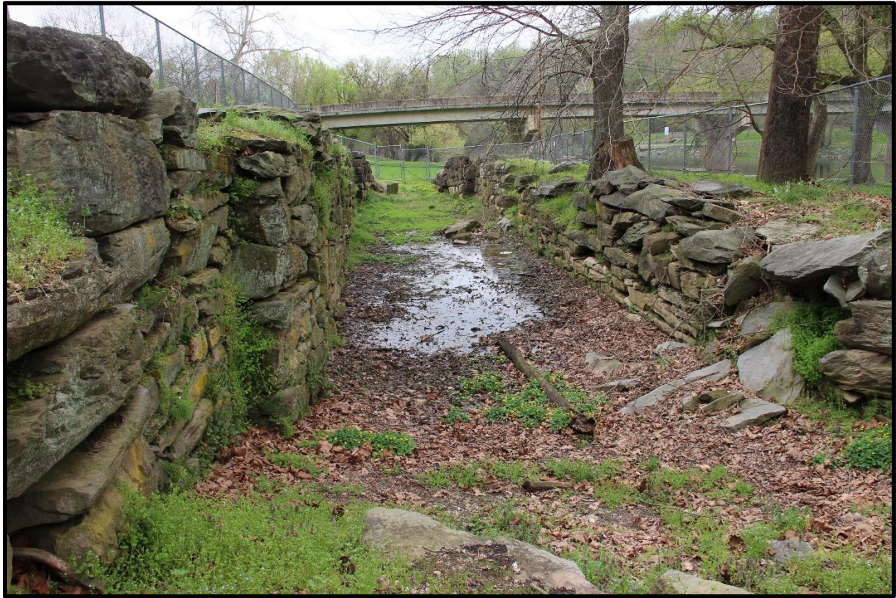
Photo 3: Detail, Conestoga Canal Lock No. 6 showing lock chamber and relationship to River Road (SR 3017) Bridge. View from northern extent of lock chamber, facing southwest.
