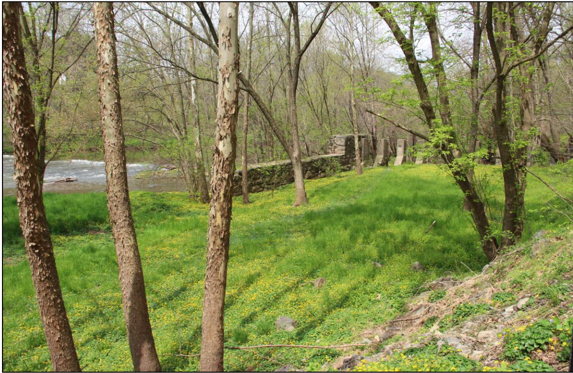
Photograph 7: Overview, Lock No. 5, showing altered west wall of lock (middle), twentieth century sluice gates (right), and remnant of demolished, twentieth century hydroelectric dam (left), facing northwest.
