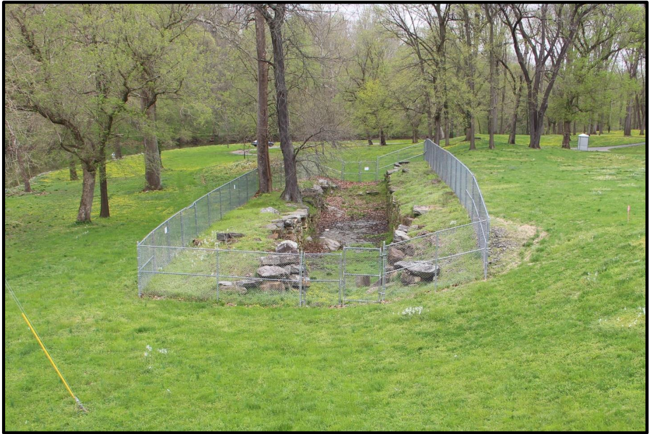
Photo 1: Overview, Conestoga Canal Lock No. 6 showing ruins of lock and security fencing. View from River Road (SR 3017) Bridge near Conestoga Boulevard, facing north.
